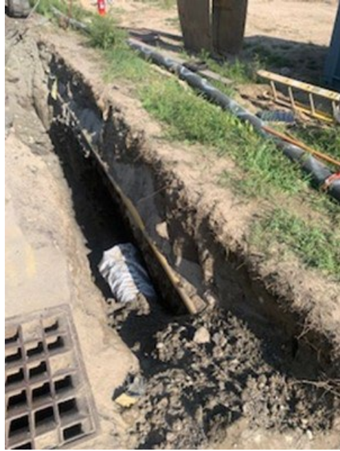
Photo 3: Exposed Gas Main along the 12-inch Water Main Alignment
