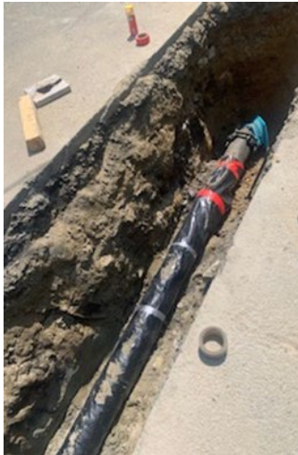
Photo 2: Water Service Connection on Auburn Street at Eliot Woods
